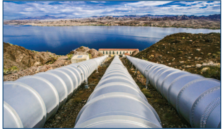
Whitsett Intake Pumping Plant on the Colorado River.
